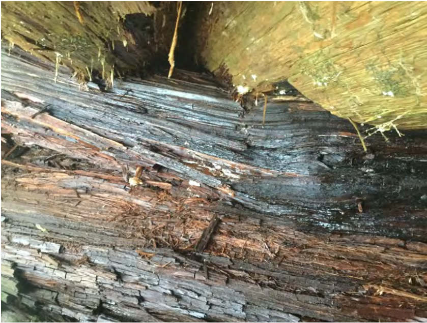
Crushed top crib log at upstream left bank
